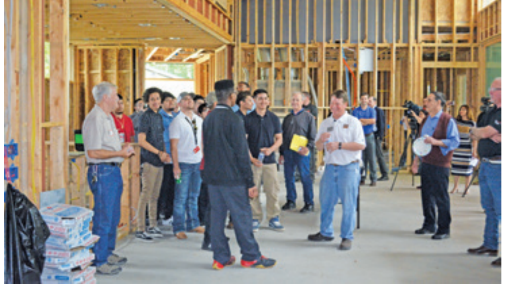
Dallas BA President Michael Turner hosts construction trades students at a jobsite tour.
