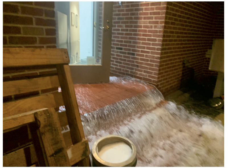
Dallas BA offices suffered catastrophic damage due to flooding caused by a burst sprinkler pipe during last winter's unprecedented icy conditions.
